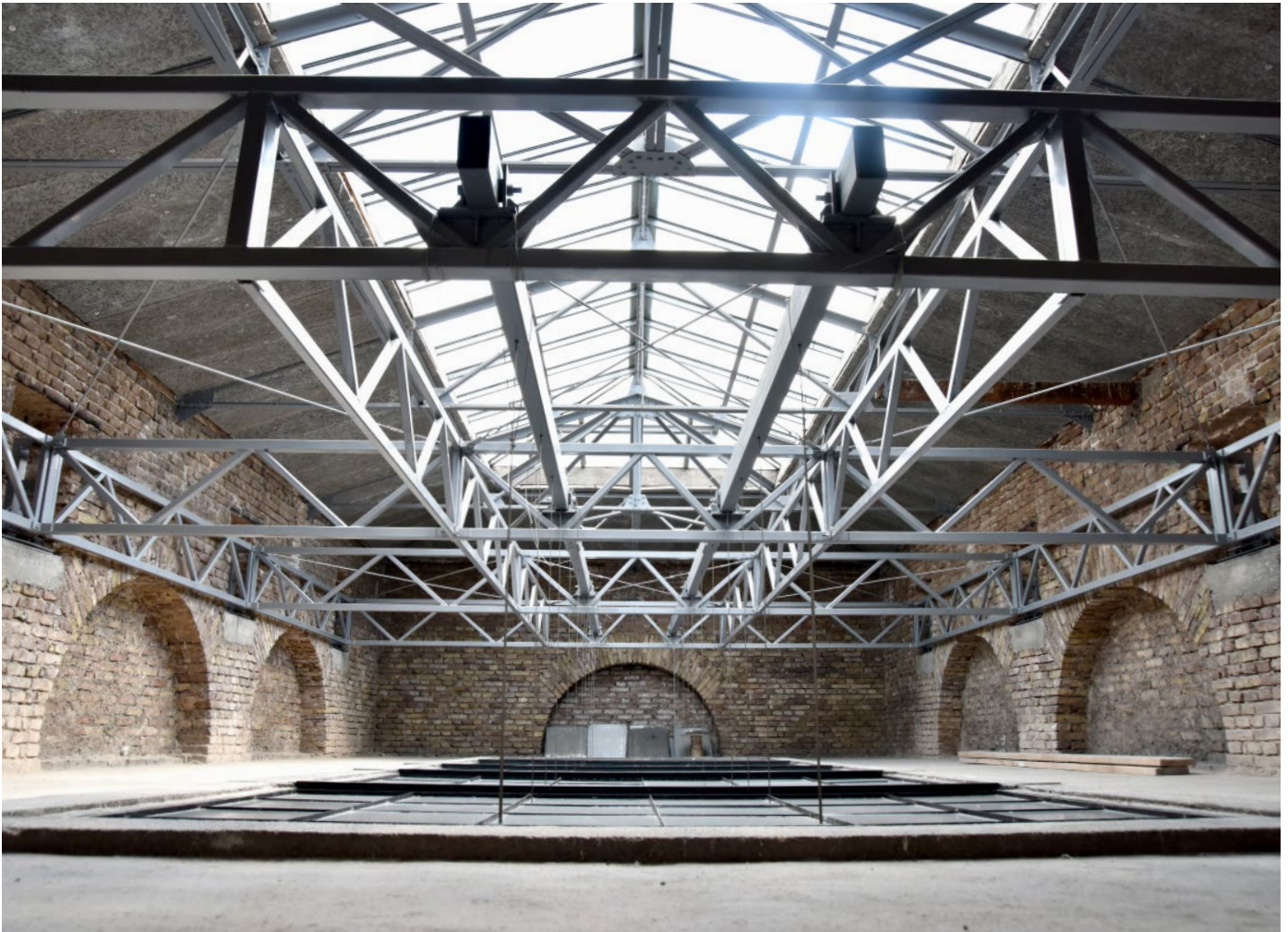
Photo 12: Restoration of the glass ceiling and the roof above the Prehistory Section, Ideologija, Sarajevo
