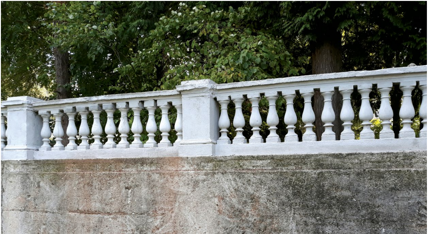
Photo 6: Restoration of the balustrade fences of the complex of the National Museum of Bosnia and Herzegovina, Commission to Preserve National Monuments
