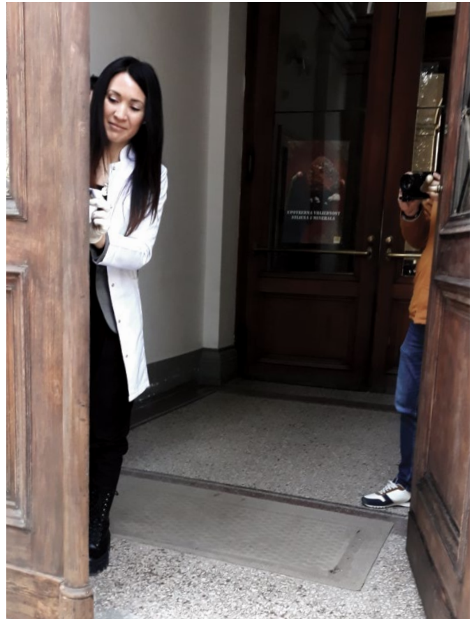
Photo 21: The partial restoration and replacement of the wooden window frames and doors, Commission to Preserve National Monuments
